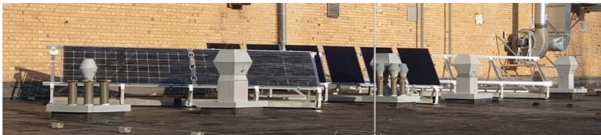
Figure 11: System with integrated PV and electrolysis modules, ready for operation
