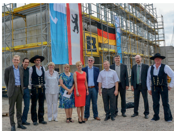
The topping-out ceremony took place on July 27, 2016, in the presence of construction firms, guest VIPs, and HZB staff.
